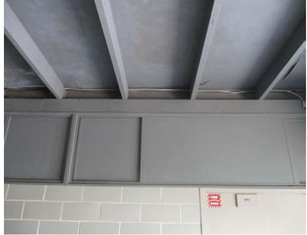
Picture 8 Building 1 - Breezeway with Wood Fill Where Glass Existed
