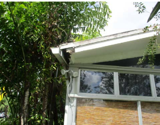
Picture 5 Building 1 - Deteriorated Roof Soffit at SE Corner
