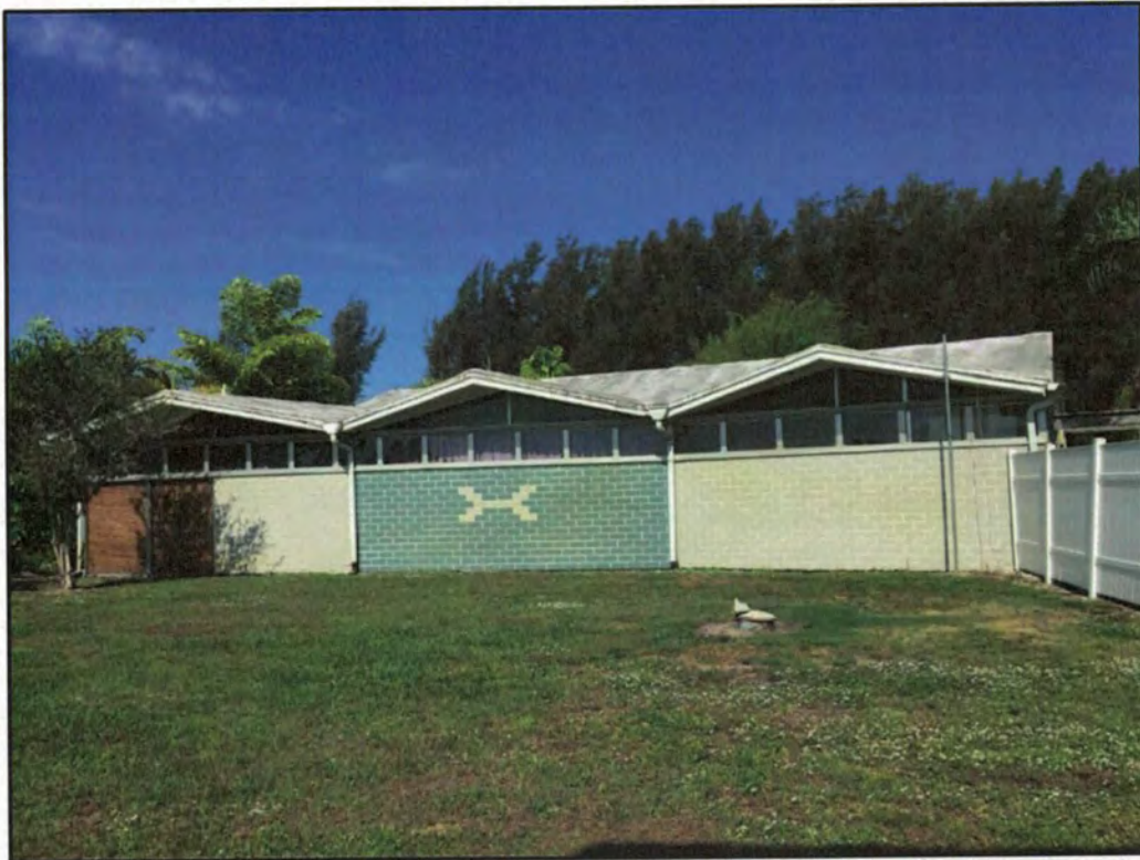
Photo 16. South structure of the Spa Building. Note the hourglass in tiles representing the shape of the springs' basin (April 2016).
