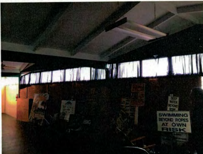
Interior of meeting room showing folded plate roof configuration with non-bearing walls and clerestory glass
