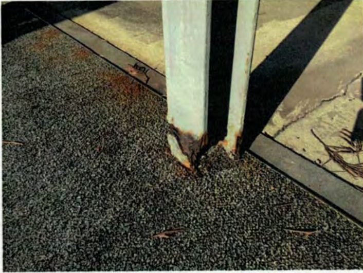
Steel columns at central promenade with deferred maintenance
