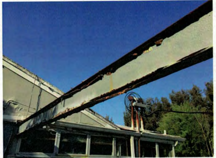
Steel beams at central promenade with deferred maintenance
