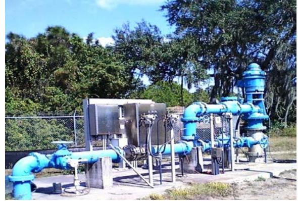
Aquifer Storage & Recovery Piping
