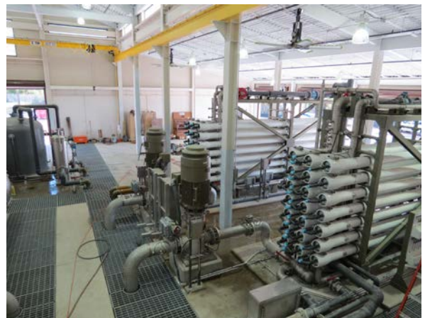
Reverse Osmosis Plant
