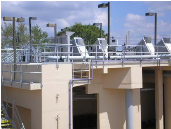
Wastewater Treatment Plant
