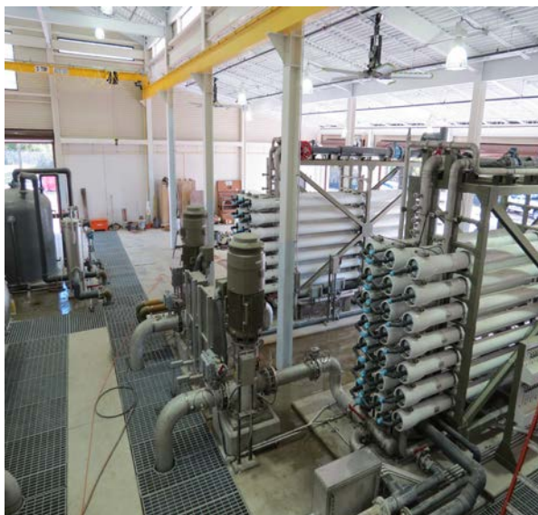
Reverse Osmosis Plant
