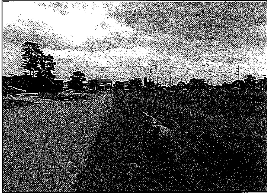
Existing Frontage Road with standing water in roadside swales
