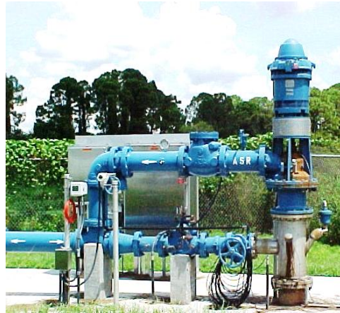
Aquifer Storage & Recovery Piping
