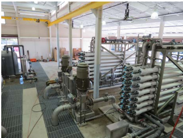
Reverse Osmosis Plant
