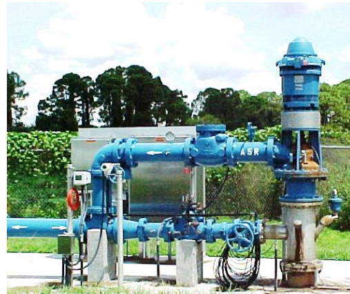
Aquifer Storage & Recovery Piping
