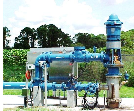
Aquifer Storage & Recovery Piping
