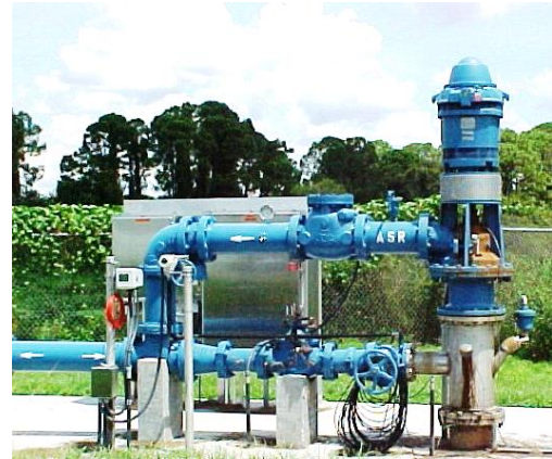
Aquifer Storage & Recovery Piping
