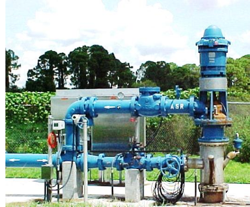
Aquifer Storage & Recovery Piping
