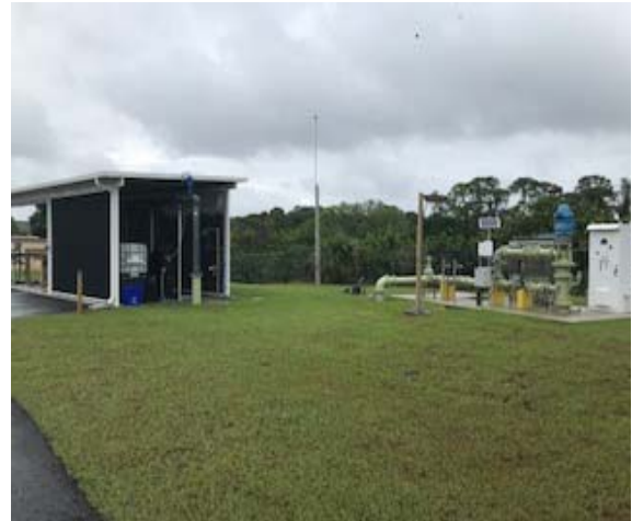
Aquifer Storage & Recovery Piping
