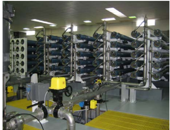
Reverse Osmosis System
