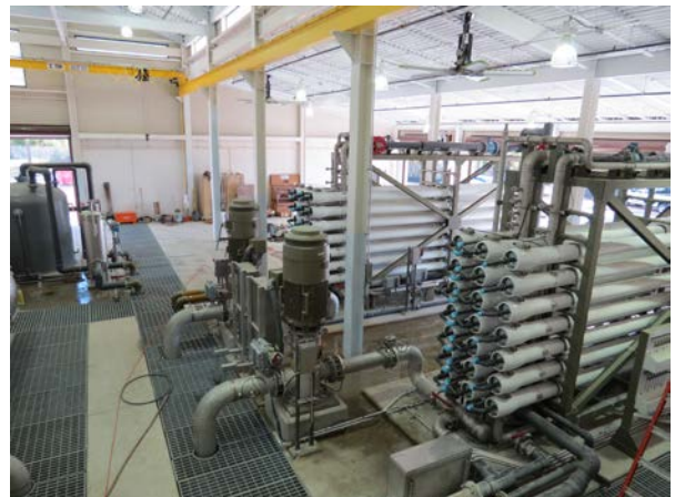
Reverse Osmosis Plant
