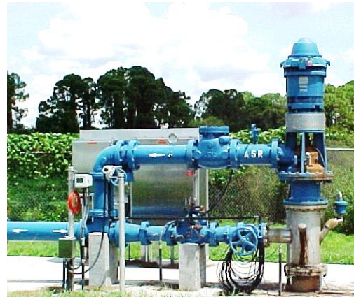
Aquifer Storage & Recovery Piping
