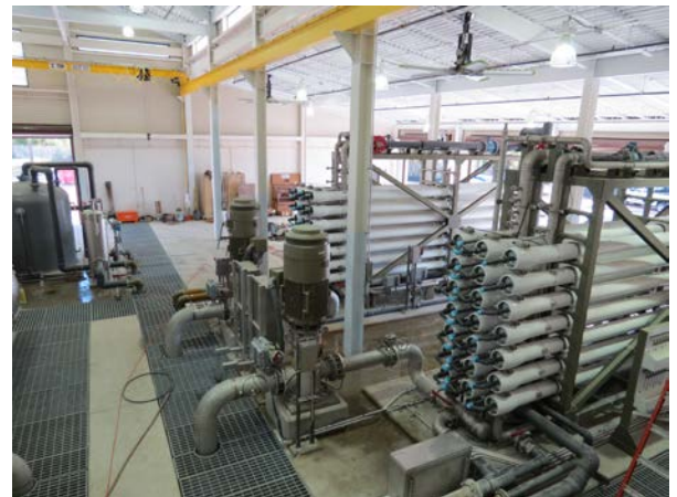
Reverse Osmosis Plant
