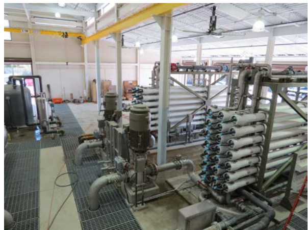
Reverse Osmosis Plant
