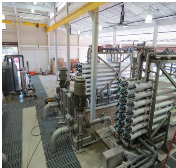
Reverse Osmosis Plant
