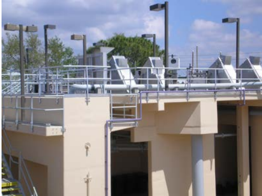
Wastewater Treatment Plant
