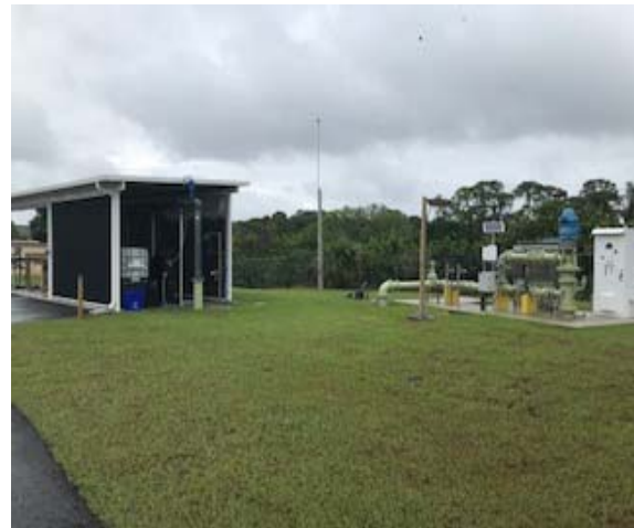
Aquifer Storage & Recovery Piping
