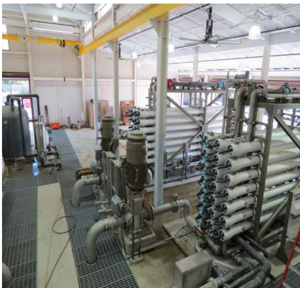
Reverse Osmosis Plant
