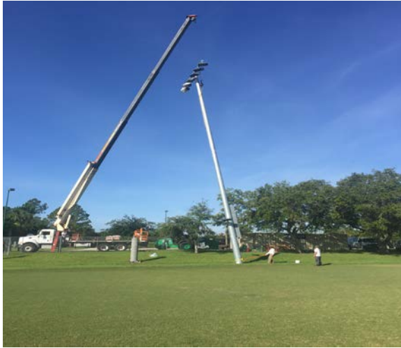
Field Lighting at Butler Park
