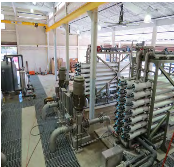
Reverse Osmosis Plant
