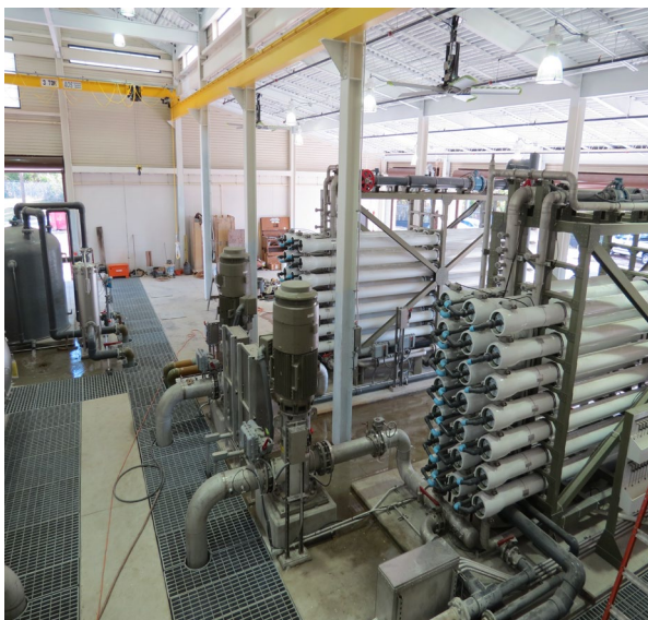
Reverse Osmosis Plant
