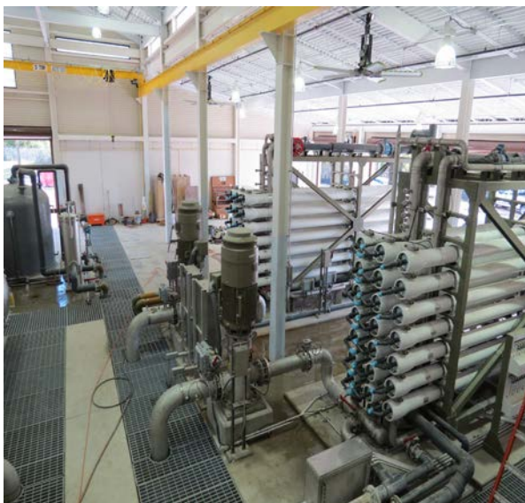
Reverse Osmosis Plant
