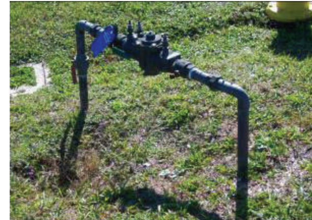
Residential Backflow Prevention Device on Water Line
