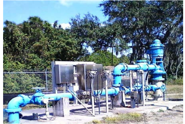
Aquifer Storage & Recovery Piping
